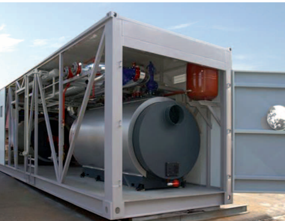
Container biomass boiler
